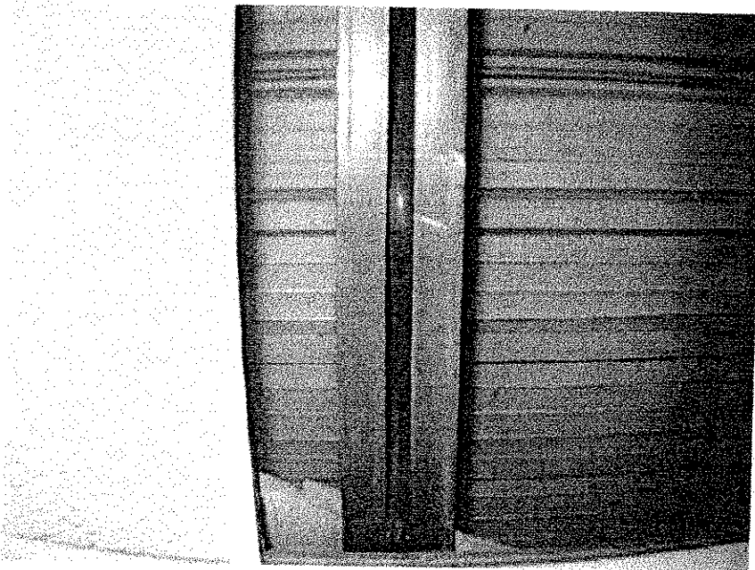
Photo 6: Non-Welded Joint Discovered at Panel Point 4 on Joist J147
